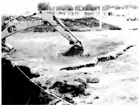
Photo 9. View north; ground cracks in yard of San Fernando Juvenile Hall. Cracks resulted from sliding and settling along wet, sandy layers of alluvium during shaking. Strongest cracks did not extend beneath floor of trench (T9). Close-up view shown in photo 10. Photo by James E. Kahle.
